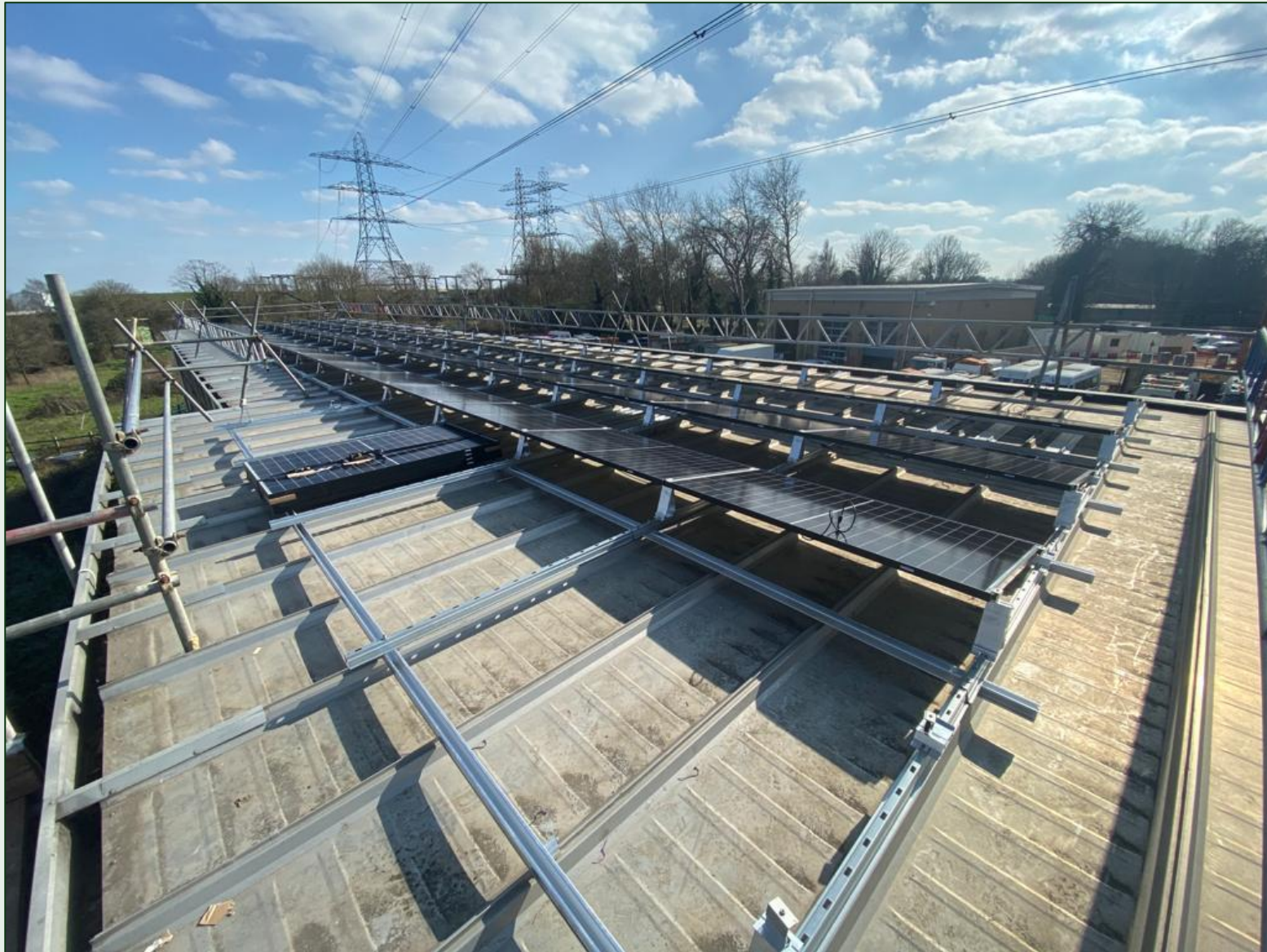
5.7. Figure 11: Solar Panels at White House Depot
